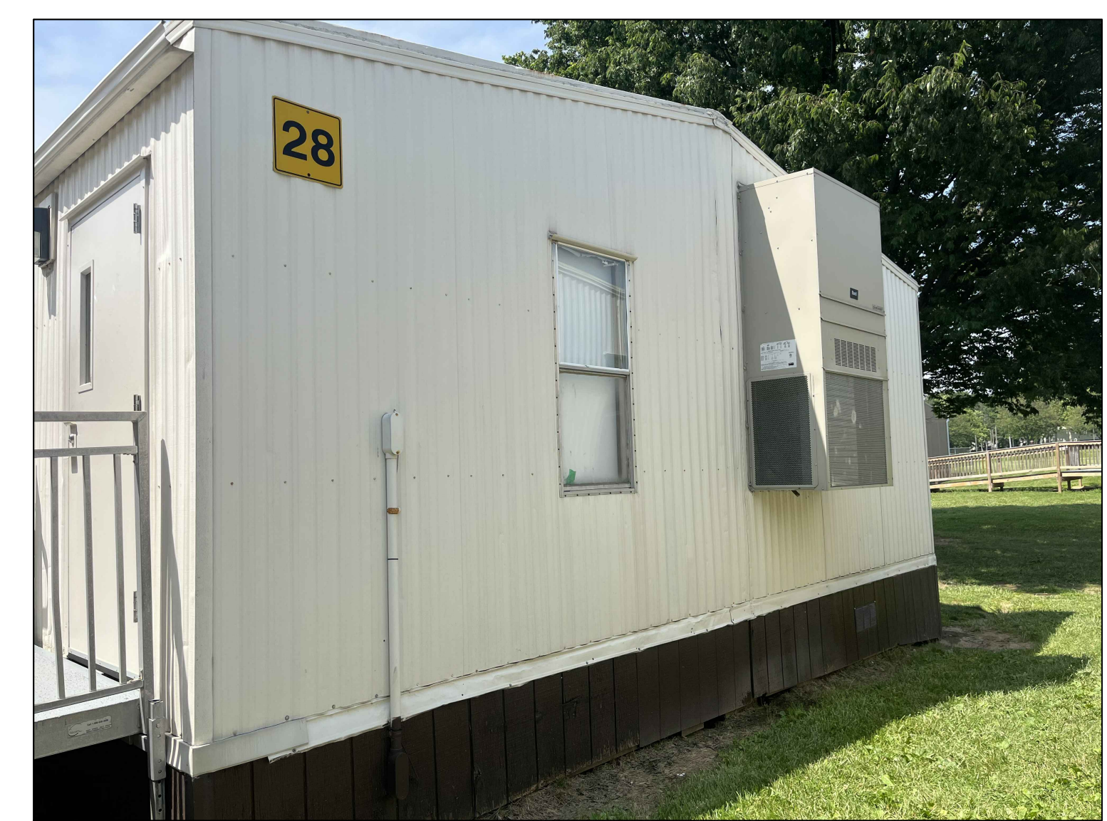
2 CRADLEROCK ES/LAKE ELKHORN MS RELOCATABLE CLASSROOM #28-EXISTING CONDITION PHOTO ME3.2 SCALE: NO SCALE
