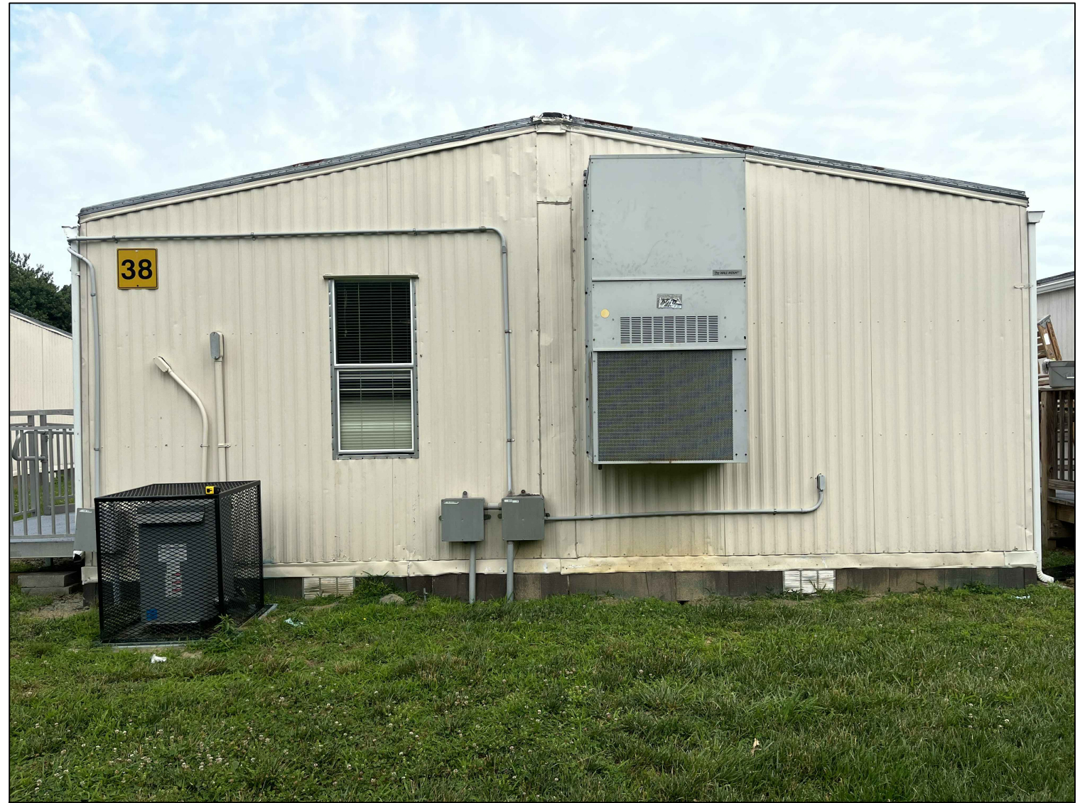
2 MANOR WOODS ES RELOCATABLE CLASSROOM #38-EXISTING CONDITION PHOTO ME6.4 SCALE: NO SCALE
