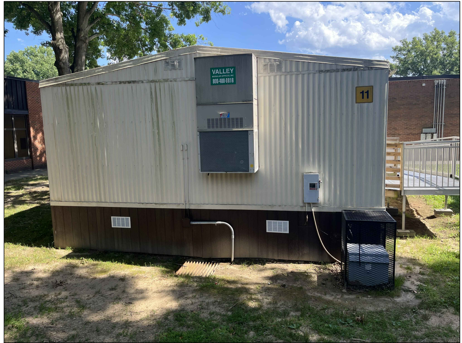
2 CLEMENS CROSSING ES RELOCATABLE CLASSROOM #11-EXISTING CONDITION PHOTO ME2.2 SCALE: NO SCALE
