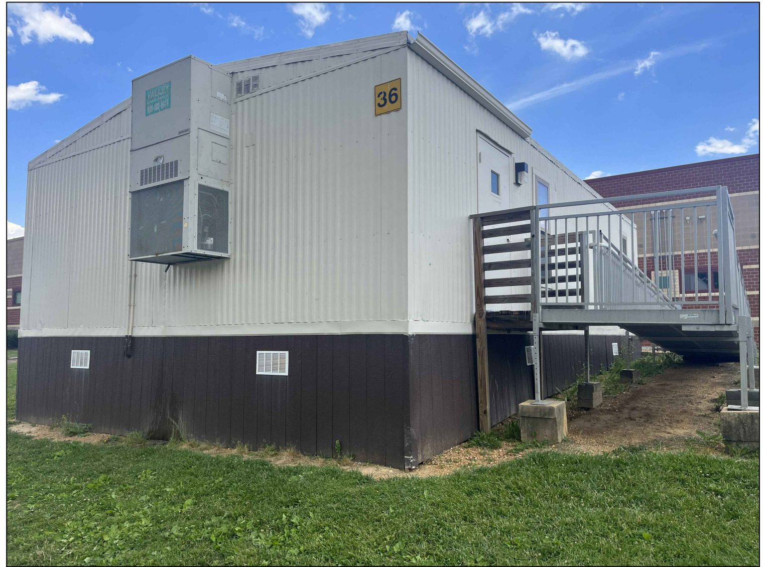
2 BONNIE BRANCH MS RELOCATABLE CLASSROOM #36-EXISTING CONDITION PHOTO ME1.2 SCALE: NO SCALE
