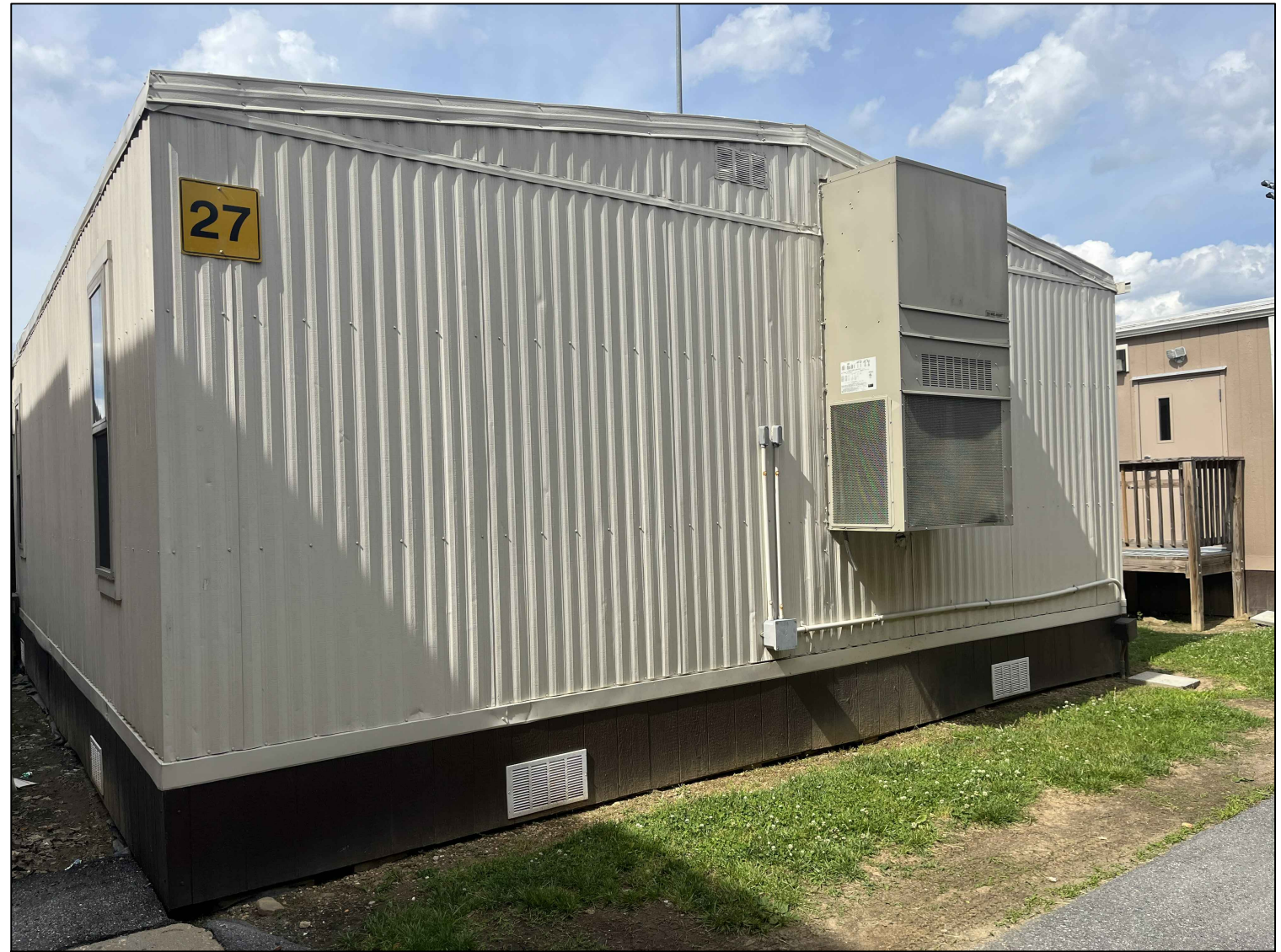
2 MOUNT HEBRON HS RELOCATABLE CLASSROOM #27-EXISTING CONDITION PHOTO ME7.2 SCALE: NO SCALE
