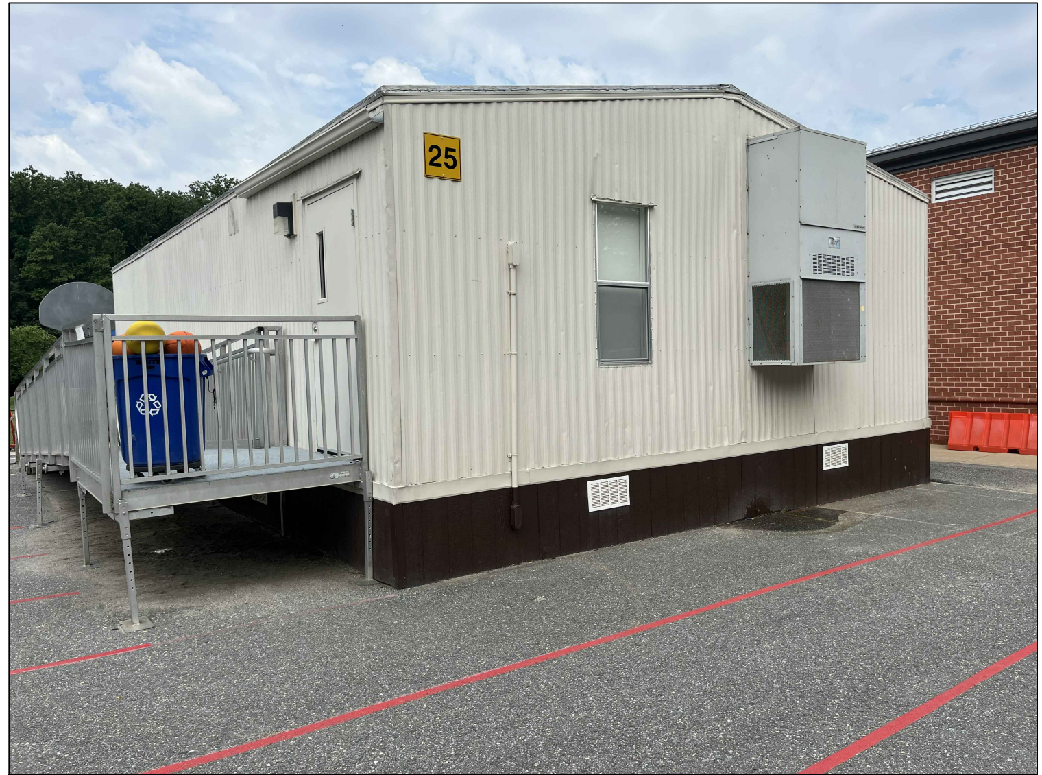
2 MANOR WOODS ES RELOCATABLE CLASSROOM #25-EXISTING CONDITION PHOTO ME6.2 SCALE: NO SCALE
