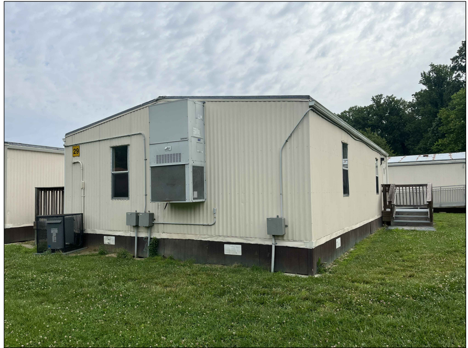
2 MANOR WOODS ES RELOCATABLE CLASSROOM #29-EXISTING CONDITION PHOTO ME6.3 SCALE: NO SCALE
