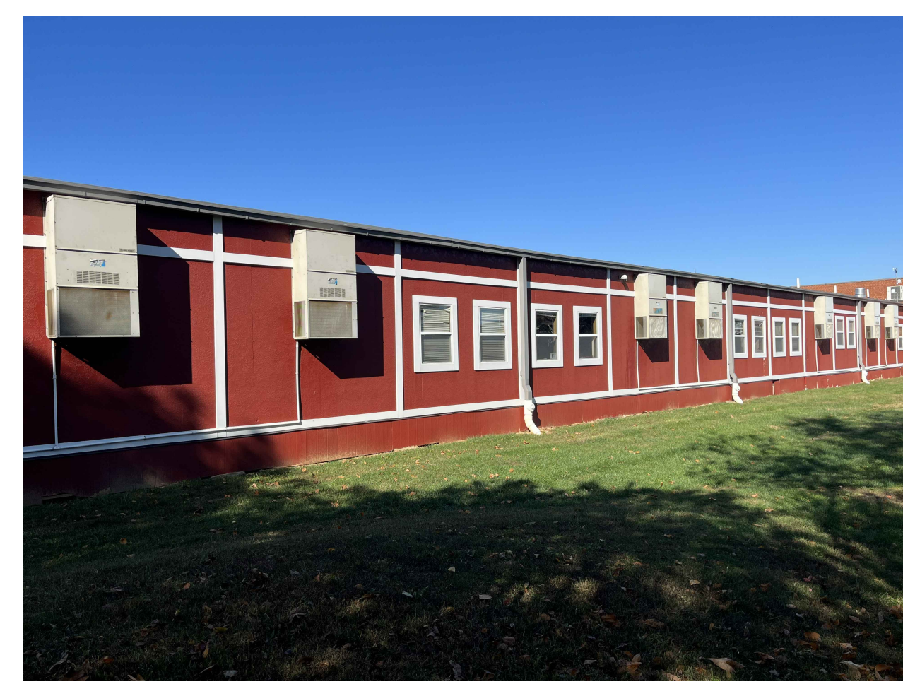
2 PHOTO OF EXISTING AC UNITS M1.1 NO SCALE
